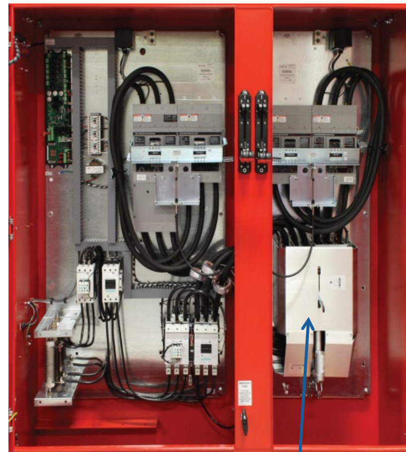
Automatic Transfer Switch
